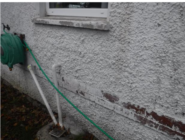
Photo 7: Detail of the south elevation of Woodbrook Side Lodge. The paint is spalling, revealing the brick string course. The cill is a concrete replacement as is the dash render
