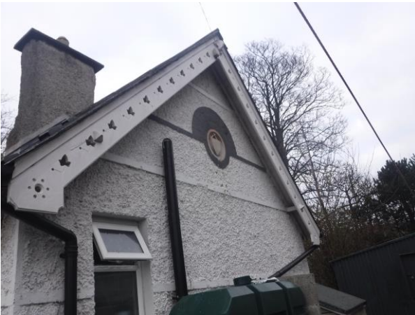
Photo 5: Detail of the east gable of Woodbrook Side Lodge showing the decorative bargeboards, brick dressings and plaque
