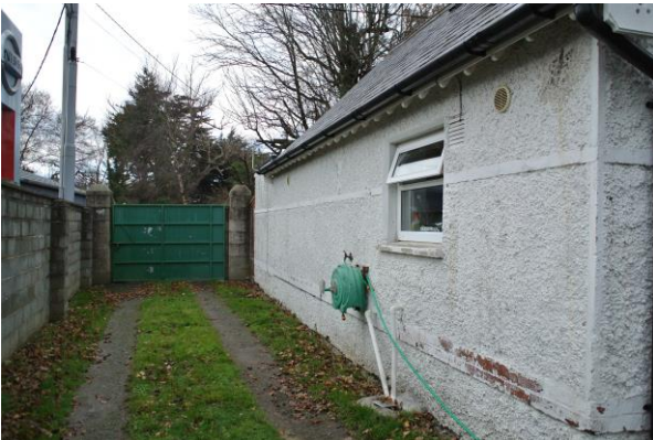
Photo 6: The south elevation of Woodbrook Side Lodge, showing the brick string courses which have been painted over. The rafters to the eaves are visible. The gutters have been replaced previously as has the fenestration and cills
