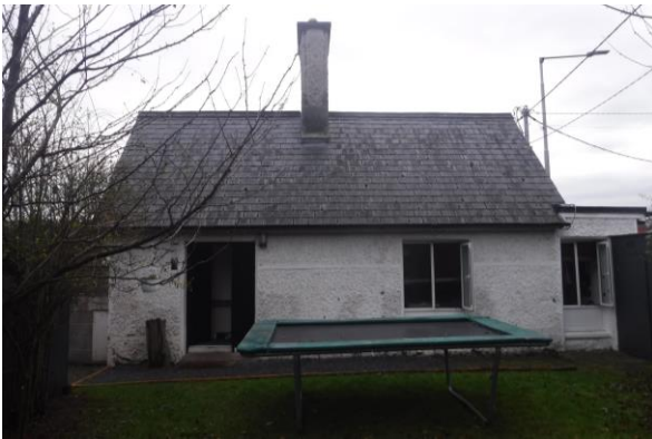
Photo 3: North elevation of Woodbrook Side Lodge showing the natural slate roof and rendered stack. The fenestration, cills and doors are all replacements
